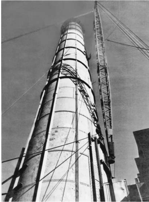
FIGURE 1.19 A 125-ft (38-m) Chicago boom mounted on a steel stack at a Consolidated Edison Company plant in New York City during alterations. Mounting provisions and installation were designed by one of the authors. (Lawrence K. Shapiro.)
